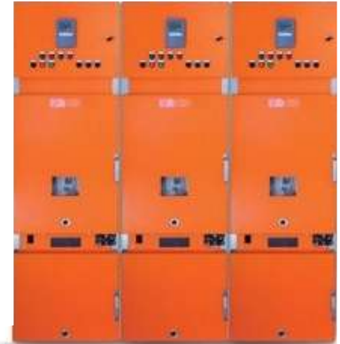
SYSclad switchboard Celds SYSclad
